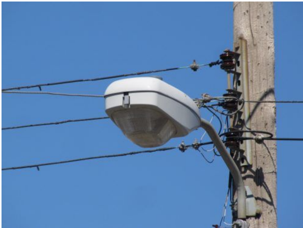
Photo 10: Overhead St. Lights
